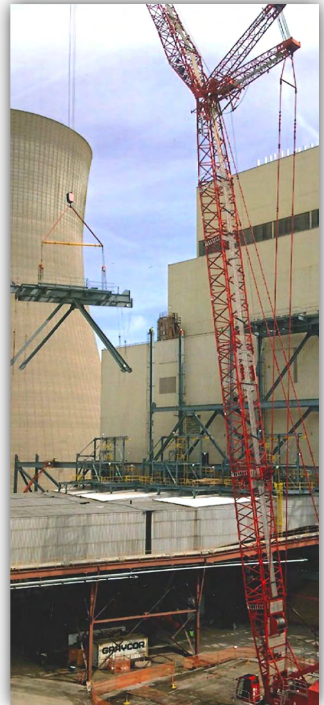
AEP Power Plant in Rockport, Indiana Manitowoc MLC-300 with 197 'Main & 177' Luffing Jib.
