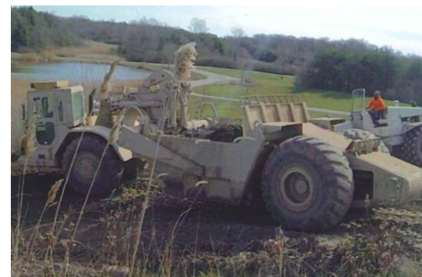
Apprentices during mandatory training hauling dirt to extend the pad for the new classroom building at Lynnville.
