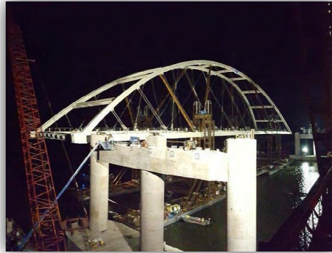
Johnson Bros. setting the bridge span on the HWY 68/80 Aurora Bridge Project in Aurora, Kentucky.
