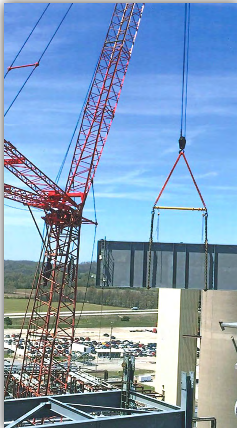
MLC-300 Manitowoc, flying in a 27 ton support beam for the new duct work on the AEP Project.
