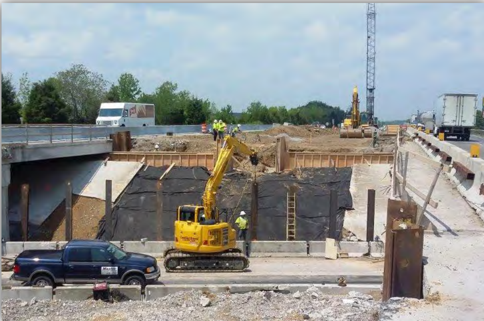
E & B Paving performing work on I-65 over Perry-Crossing Road between Sellersburg and Memphis, Indiana.
