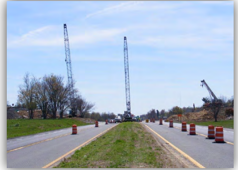
Jim Smith Contracting, LLC performing bridge work on HWY 80 in Mayfield, Kentucky
